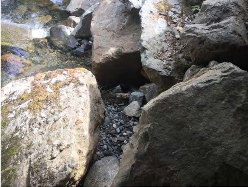
Eroding riprap at downstream right bank
