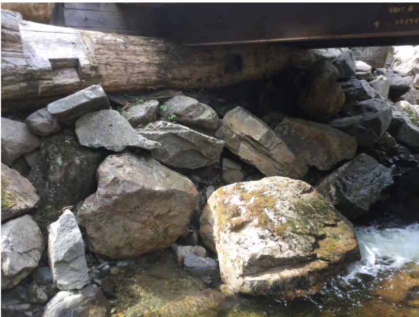
Eroding riprap right bank
