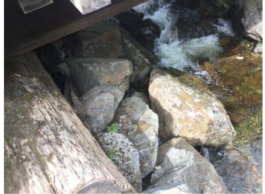
Eroding riprap at downstream right bank
